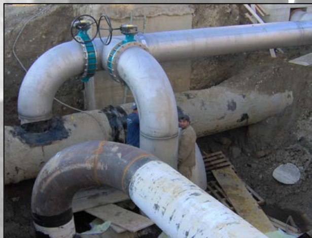
Posa in opera di tubazioni interrato DN800. Laying of Piping DN800 Buried.
