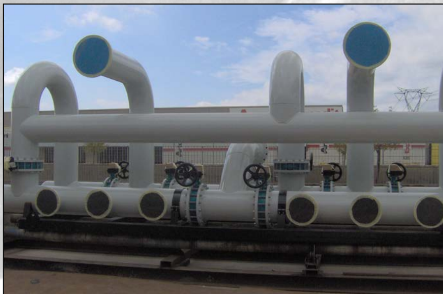
Skid DN400 precostruito ed assemblato in officina. Skid DN400 Prefabricated and assembled in work shop.
